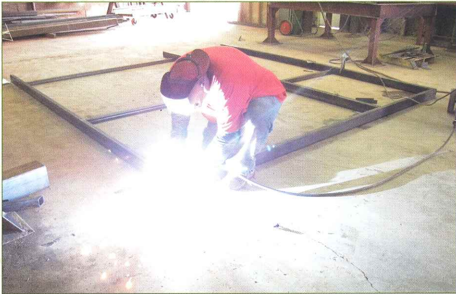
Workers at Independent Steel Company of Brooks, Ky. fabricating the support structure for Yew Dell's new entrance gates. The gates were designed by deLeon and Primmer Architecture Workshop in Louisville, also designers of Yew Dell's award-winning bank barn and pavilion.
