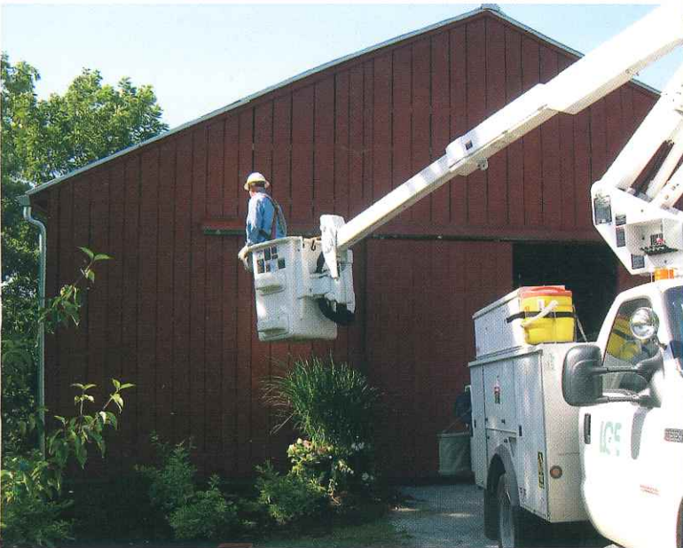
LGE's staff came complete with all the heavy equipment needed to make the painting job a snap!
