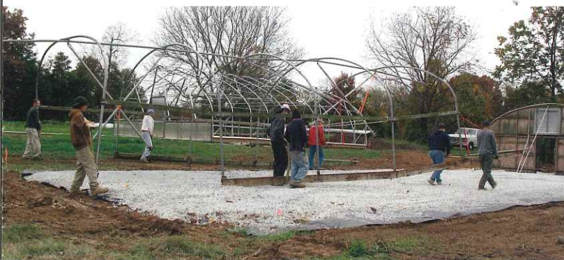
Kiel Thomson Company workers and Yew Dell volunteers literally picked up and carried away the old hoop house to make room for greenhouse construction.
