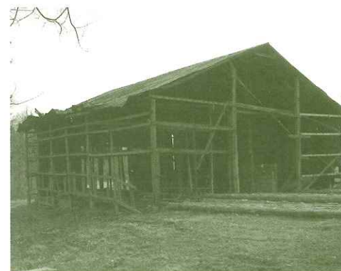
The Red Tobacco Barn at Yew Dell Gardens is under restoration. Join us for our open house on June 13 for the unveiling.
