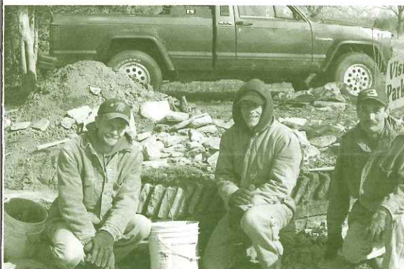
The Rock House at Yew Dell Gardens served as a loading dock for the nursery. Built in 1957 with fieldstone and Klein's signature millstone in the facade, it is flanked by two small book stacked stone walls. The stone walls are being rebuilt by Jody Edgerton, a fifth generation stone mason. The Edgerton Family's work can be traced back to 1851 at the Crestwood Baptist Church. Edgerton hopes his son will follow in his footsteps and make this family tradition six generations. Pictured (l-r) are Jody Edgerton, Bob Ash and Mark Handlon.
